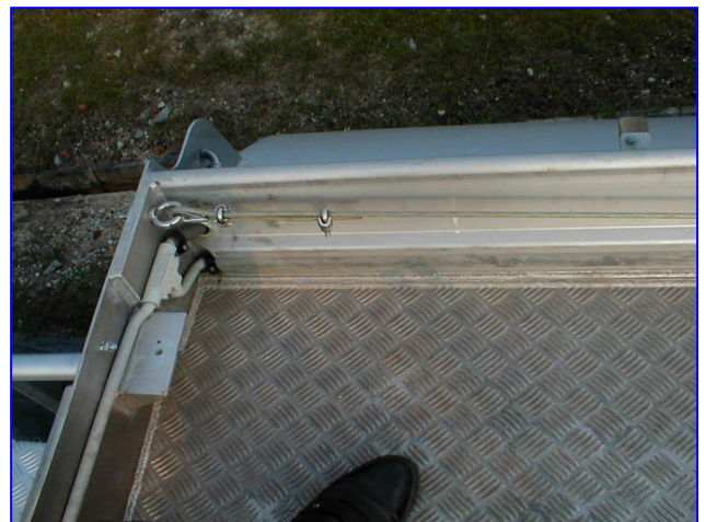
Wire-rope for safety harness on 2 sides of the cat-walk
